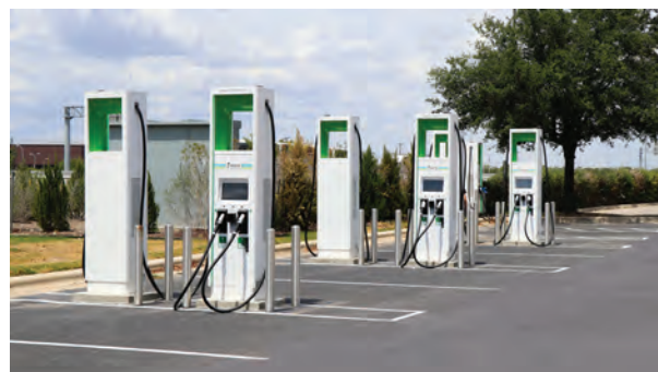
Electric vehicle charging stations at Round Rock Premium Outlets
