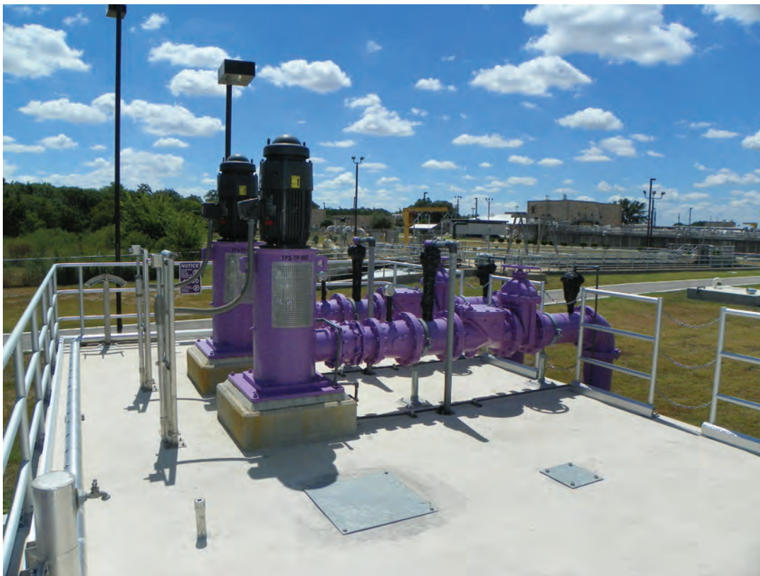
Water reuse infrastructure at Old Settlers Park
