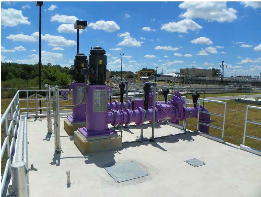
Water reuse infrastructure at Old Settlers Park
