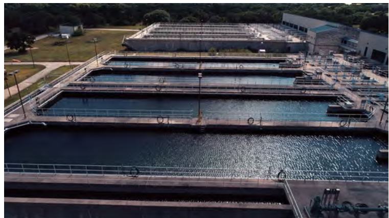
Round Rock Water Treatment Plant
